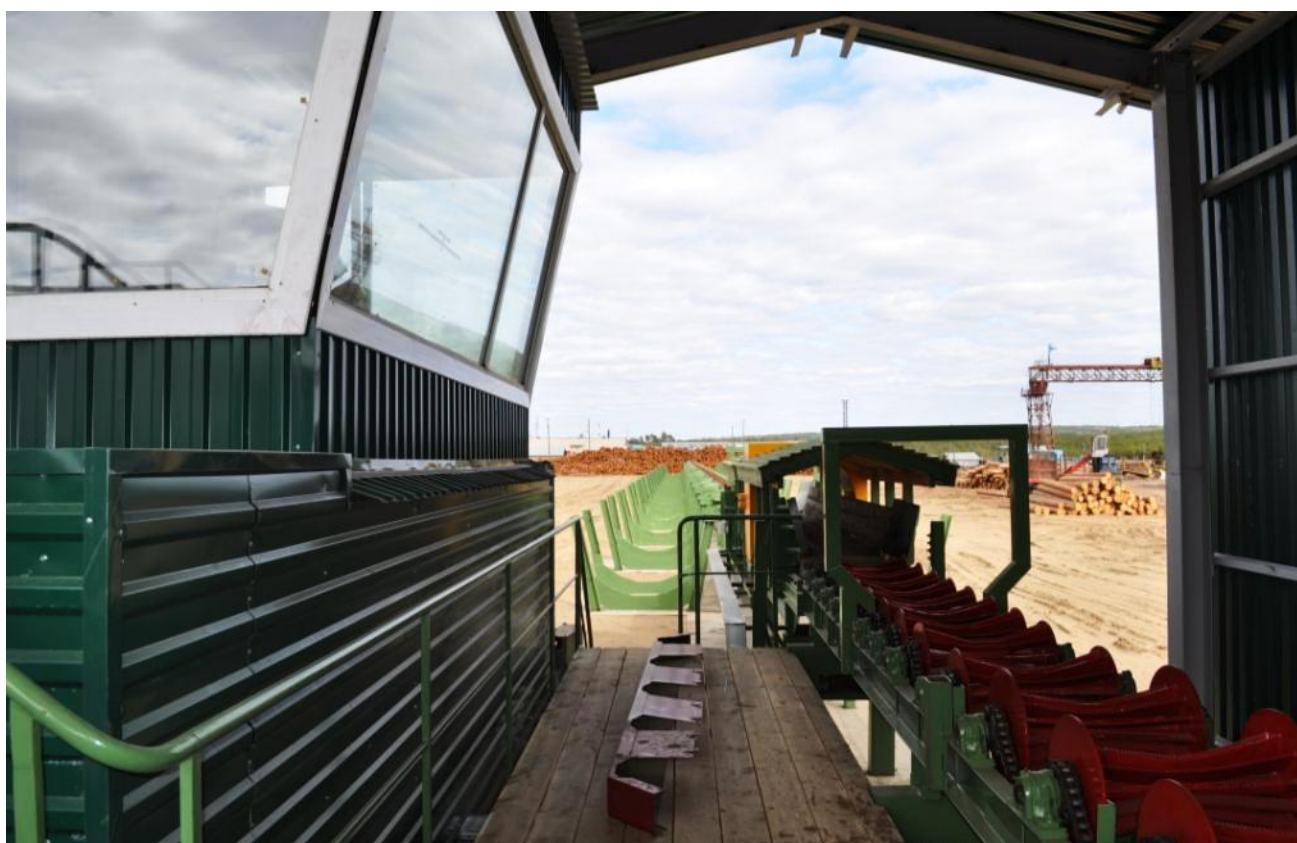
Boguchany newly erected log sorting line
